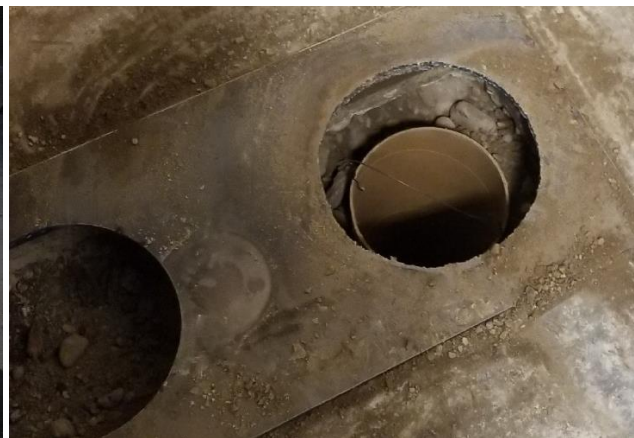
Photo#4 Shows fill below concrete pad
