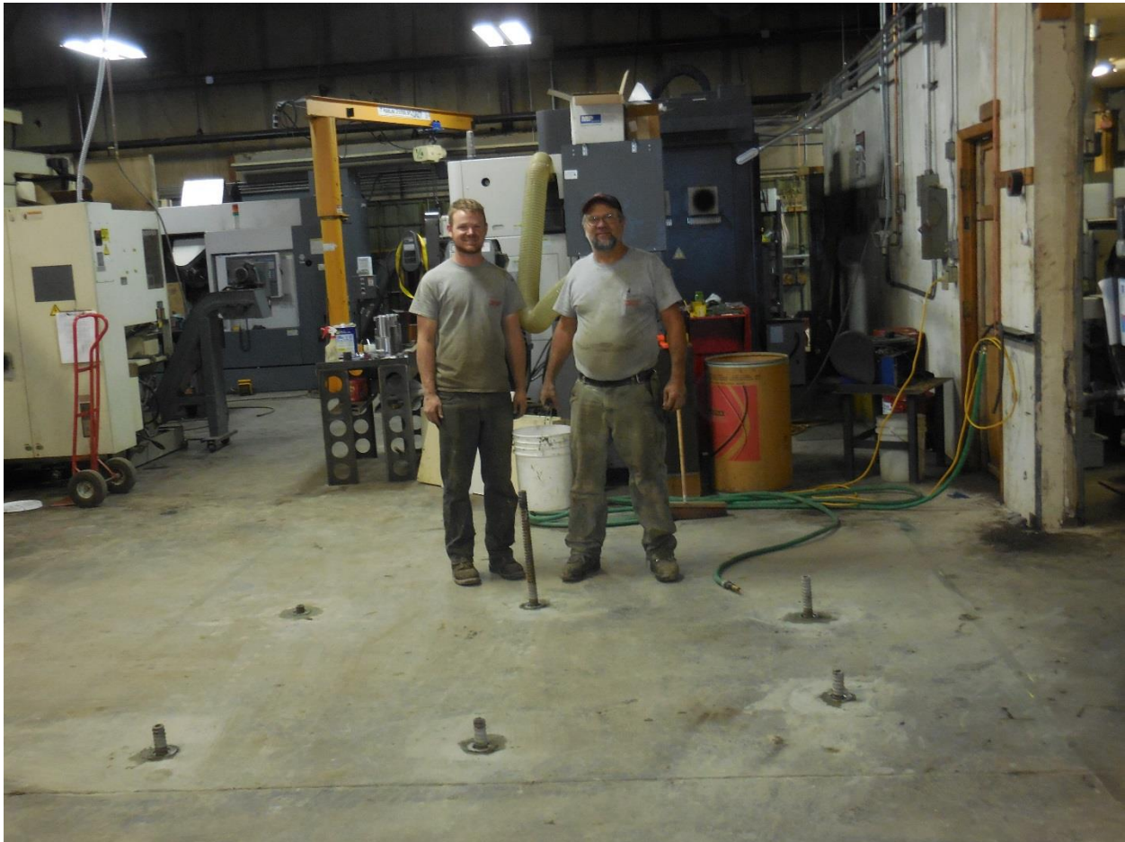
PHOTO#14 Finished micropiles for Vertical mill with proud workers, finished in one day.
